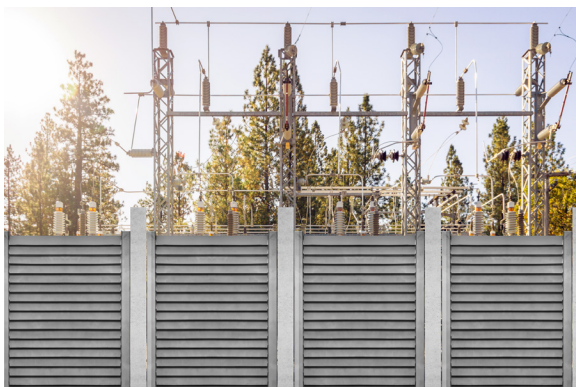
Protected substation with Ballistic Fence filling gaps between concrete dividers.
