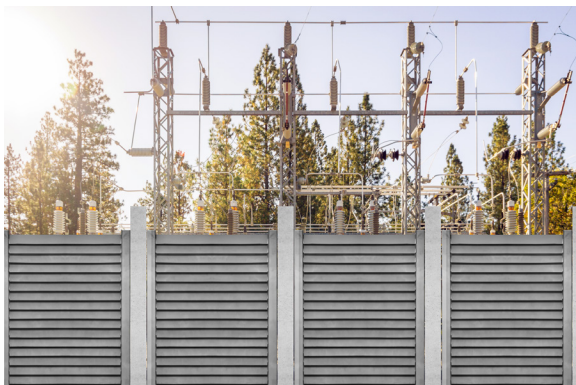
Substation with Ballistic Fence filling gaps between concrete dividers.
