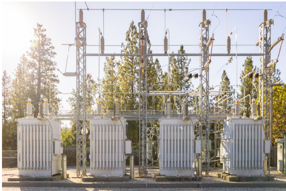
Unprotected substation leaves high cost transformers and other equipment exposed.
