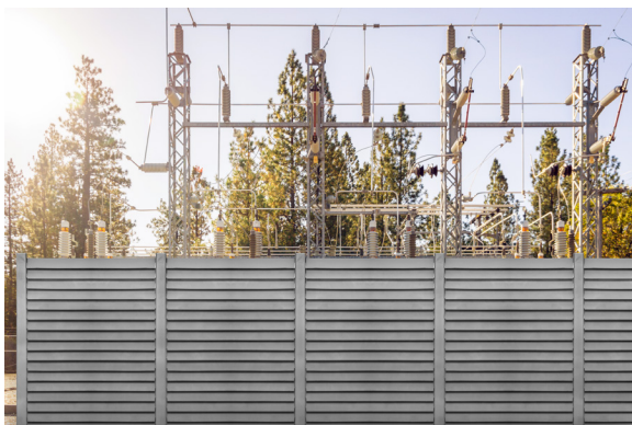
Substation with Ballistic Fence. Height and width of fence sections made to order.
