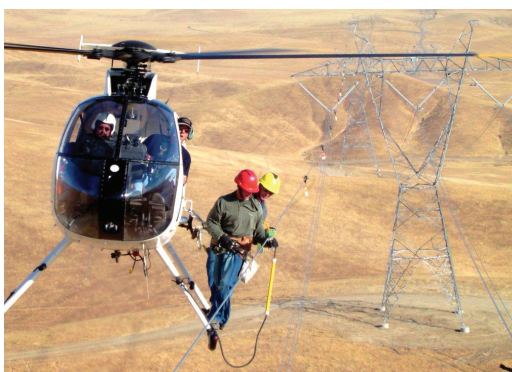
FireFly FF can be installed by helicopter
